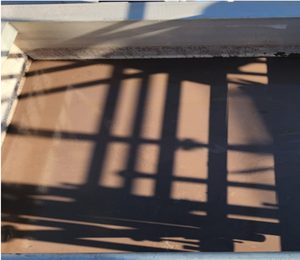
Figure 4: Muddy surface of Opal's SWTP Clarifier due to the filamentous bulking @ 203 mL/g SVI30.
