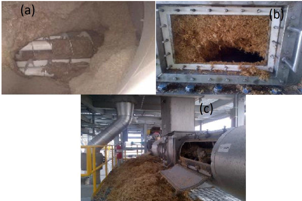
Figure 3: Corn stover bridging in a) storage bins, b) drop chute, and c) jamming in a screw conveyor.
